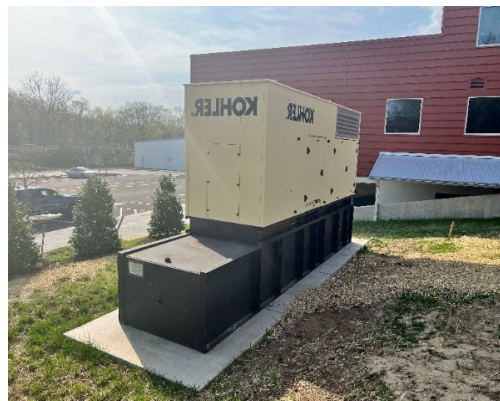
18 – Site Service Generator #2
