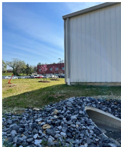
20 – Storm Outfall (To Bioretention Forebay)
