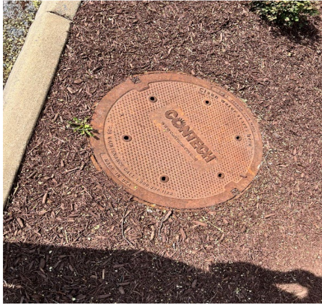
16 – Hydrodynamic Separator (Proximate to Fueling Canopy)
