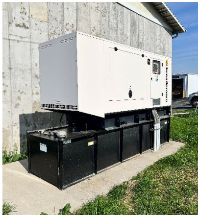
17 – Site Service Generator #1
