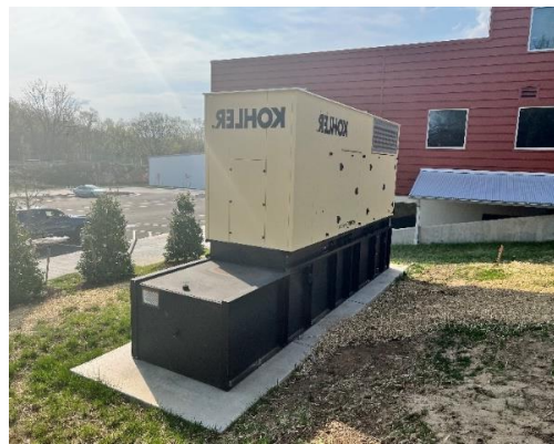
18 – Site Service Generator #2
