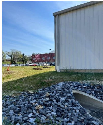
20 – Storm Outfall (To Bioretention Forebay)
