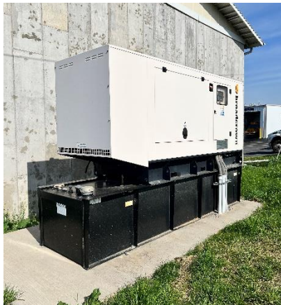
17 – Site Service Generator #1
