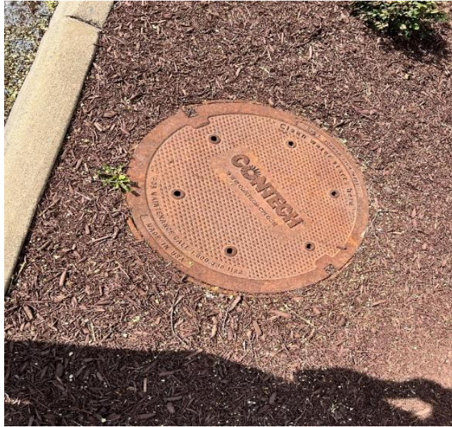
16 – Hydrodynamic Separator (Proximate to Fueling Canopy)
